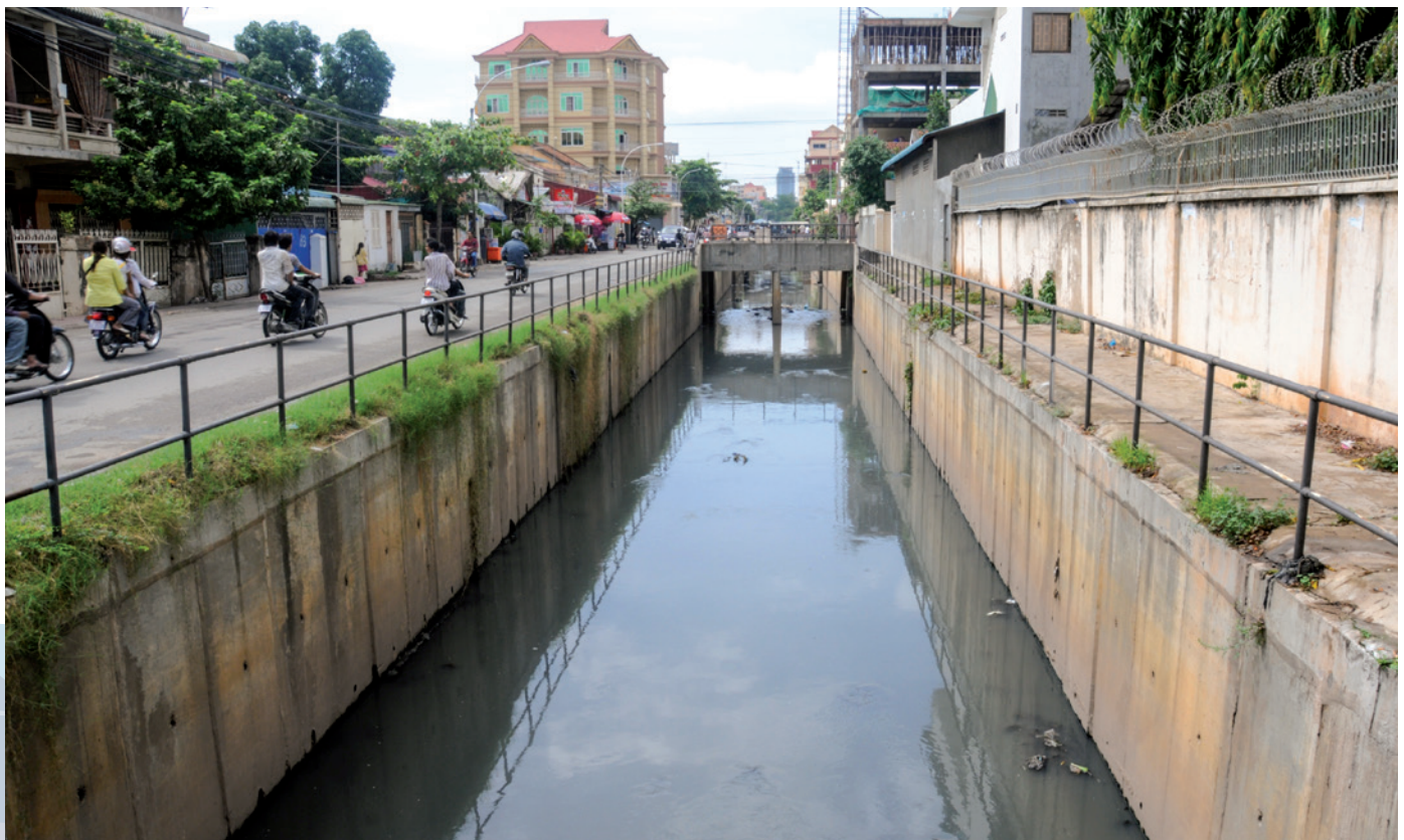
Open Sewer in Phnom Penh
