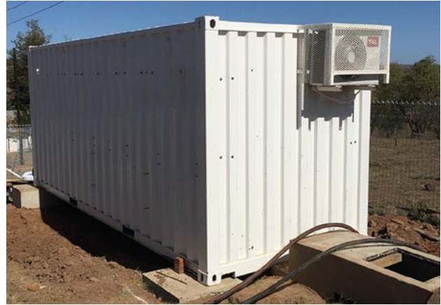
Figure 32: Minigrid system container
