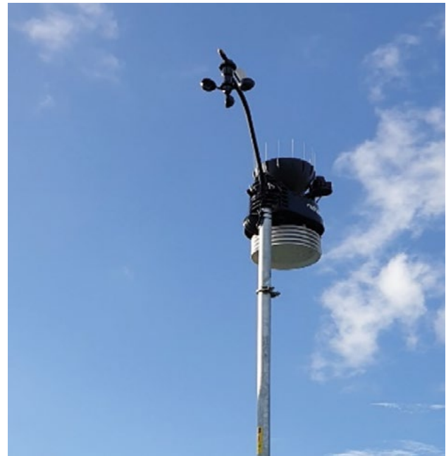
Figure 39: Minigrid on-site weather station
