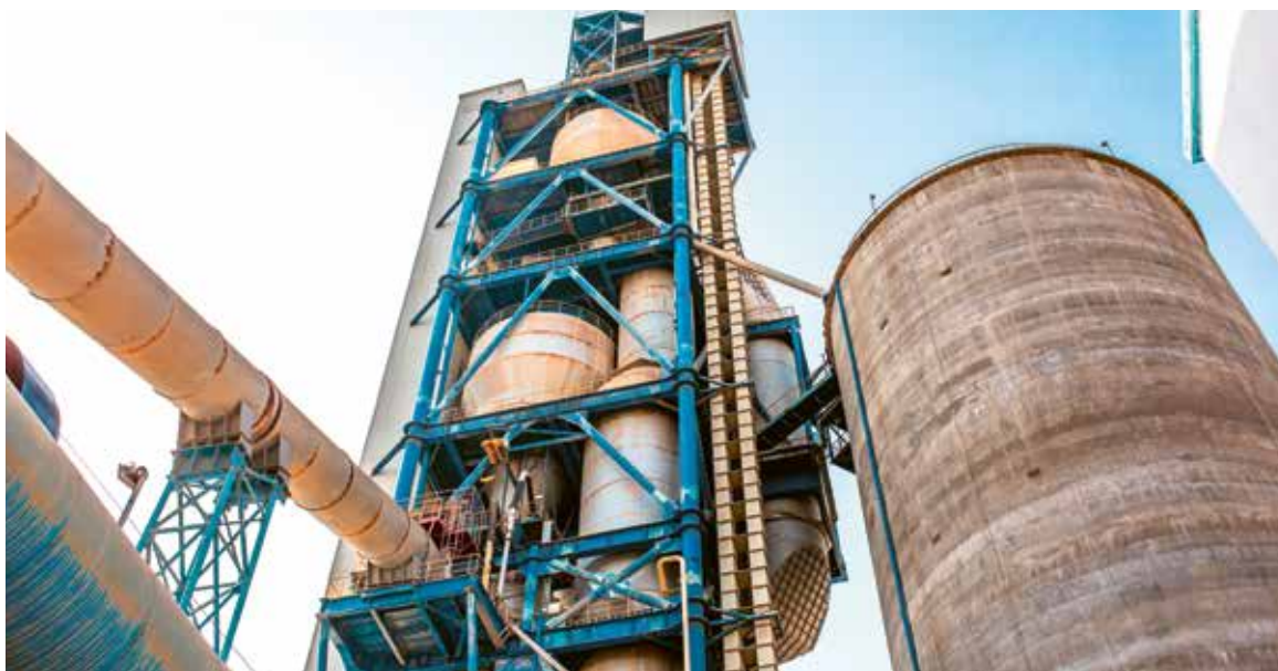
Photo: Cooling and scrubbing of exhaust gases in suspension preheater.
