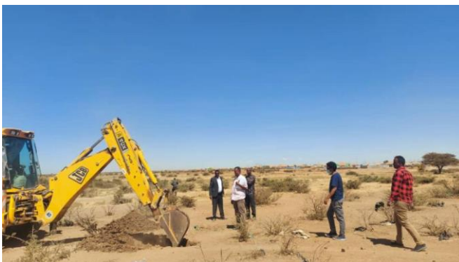
Constructions have started for the new Migration Response Center near Tog-wachale. ©IOM
