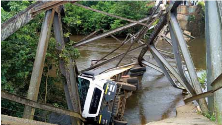
Broken bridge in Liberia.
