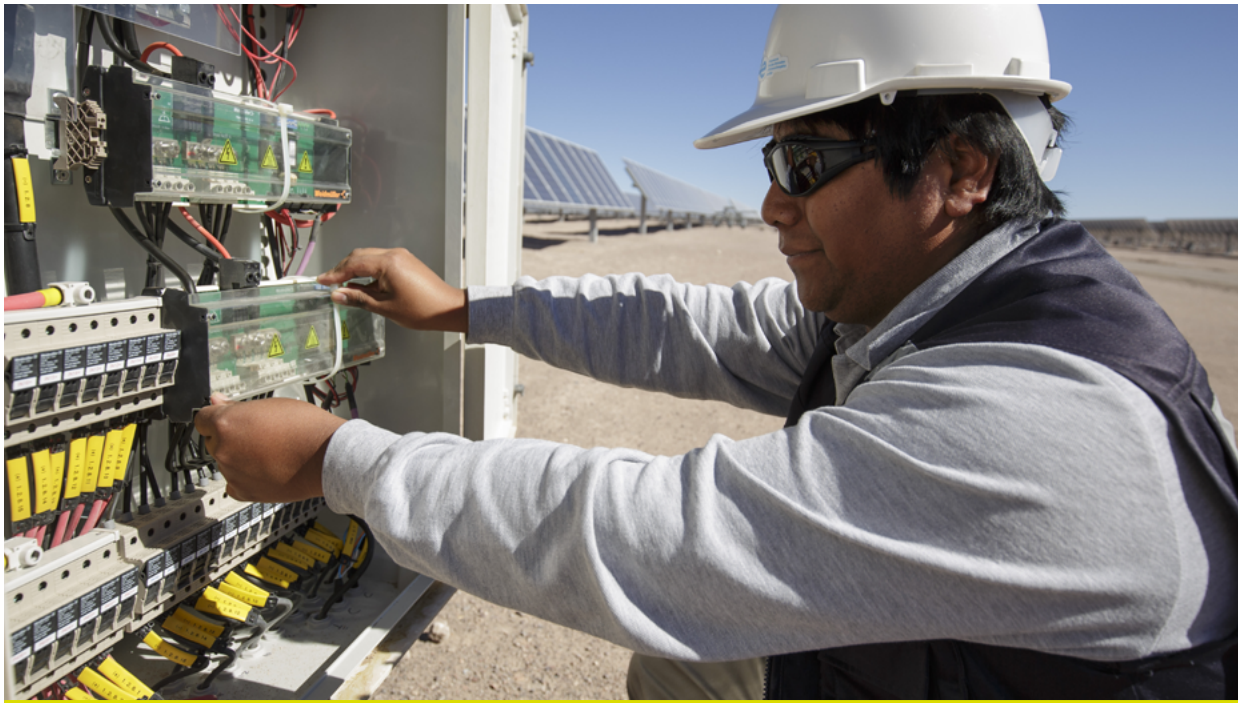
The manager of a solar plant inspecting this investment project in the Atacama Desert, Chile.
