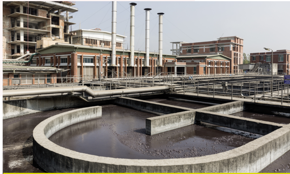
The development impact of investments is key for IPAs to understand, including the environmental characteristics. This photo shows a sewage plant for textile production in Bangladesh.
