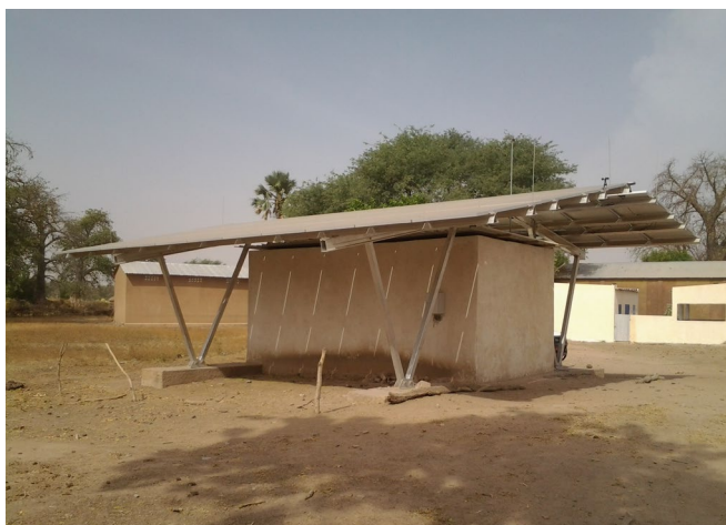
Solar mini-grids installed in a rural area, Senegal, © by Ousmane Fall Sarr
