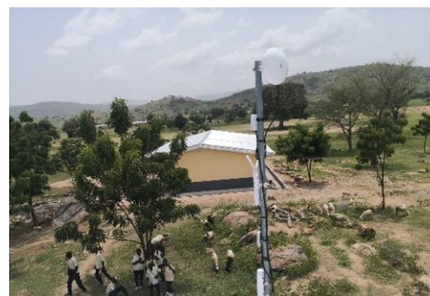
WIFI access point installed in a Mandama school
