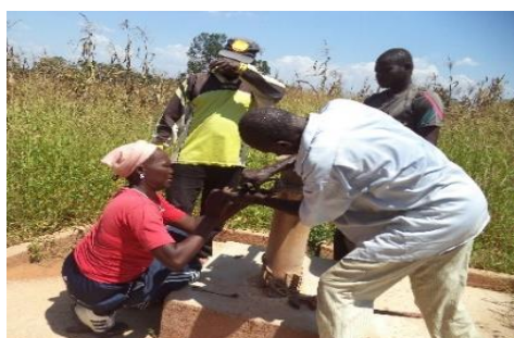
Access to drinking water and maintenance of infrastructure: repairing a water point
