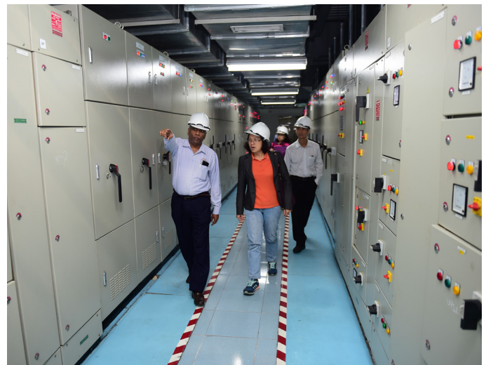
Operating system at the biomass power plant in central region of Viet Nam Photo: © GIZ
