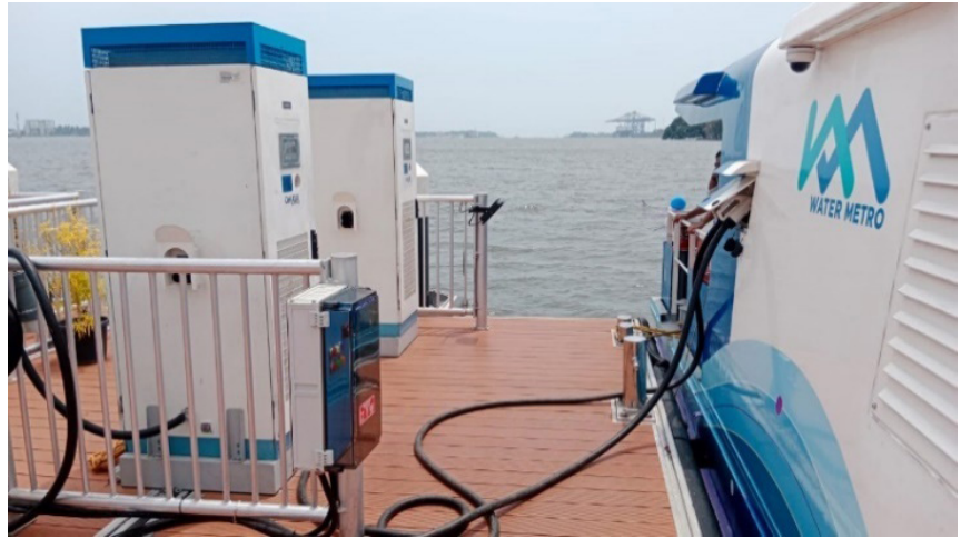
Ferry charging at Kochi Water Metro Terminal, Source: Kochi Metro Rail Limited (KMRL)/Sajan John
