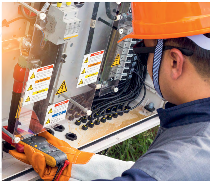
Engineer checking solar cell electrics.
