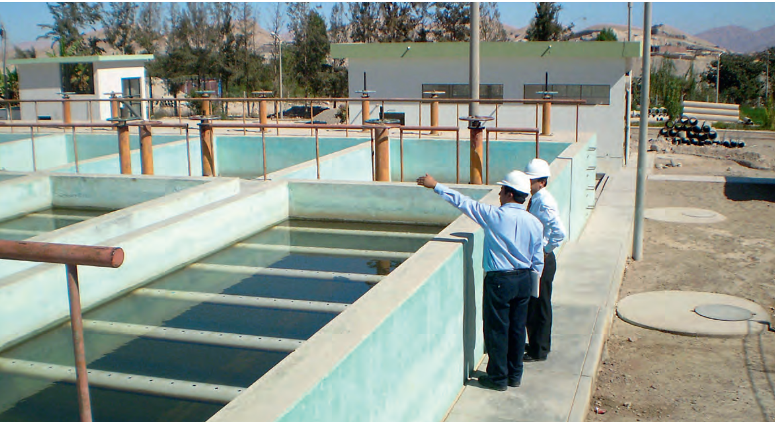
Drinking water and sanitation programme PROAGUA Peru | Demand for clean drinking water and sustainable, environmentally sound wastewater disposal is constantly growing.
