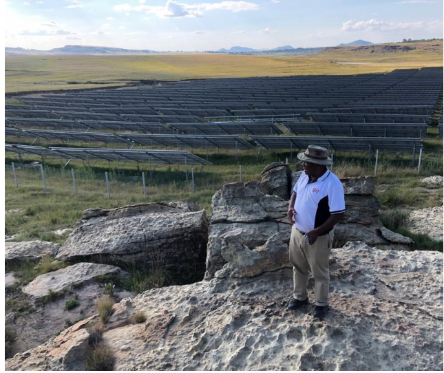
The solar farm
