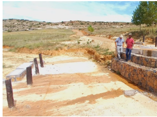
Drifts and stormwater disposal
