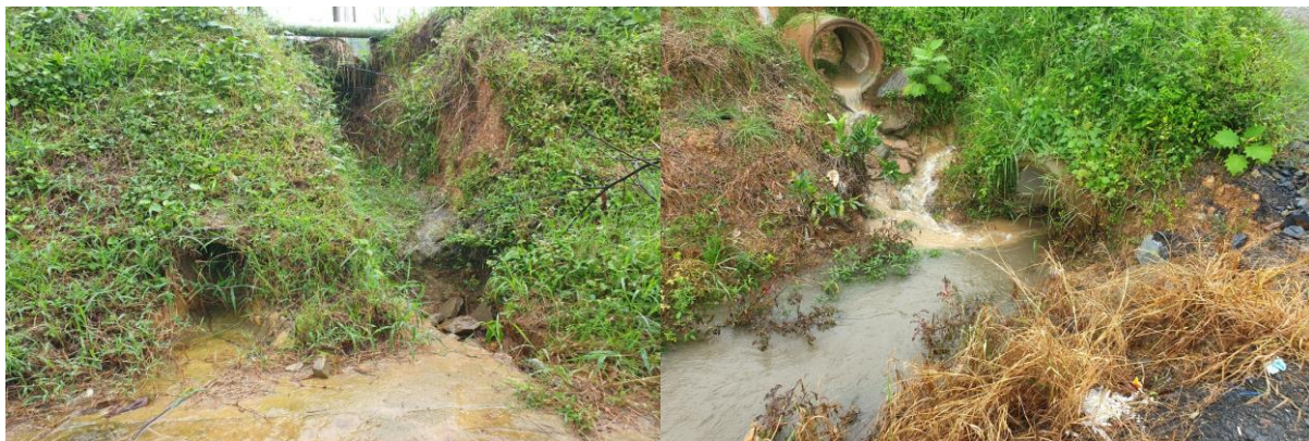
Figure 4: Examples of required drainage improvements (Highway 317 (L), Highway 3193 (R))
